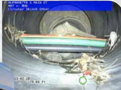
VIDEO PIPE INSPECTION VIDEO AND REPORTS
